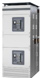
3WA incoming feeder panels
